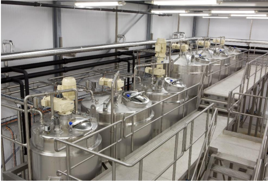
Tank & Reactor Area
