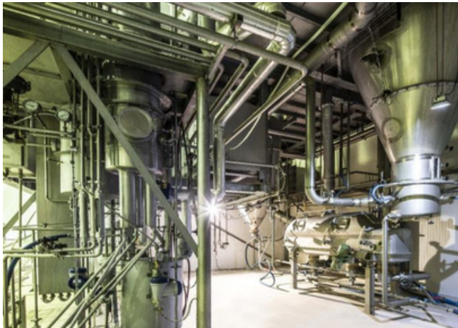
Spray dryer with internal & external fluid Bed
